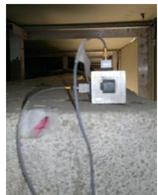
Accelerometer fixed on a beam
